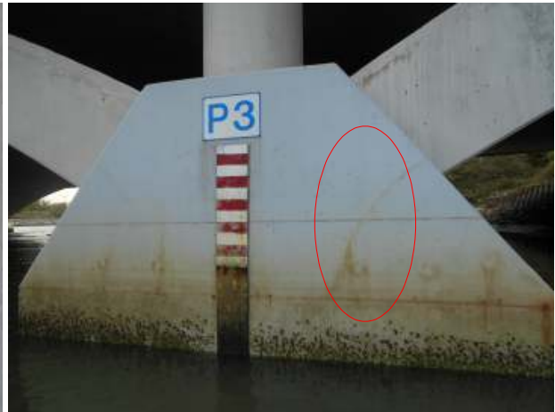
P3 교각 균열(CW=0.2mm, L=2.0m)
